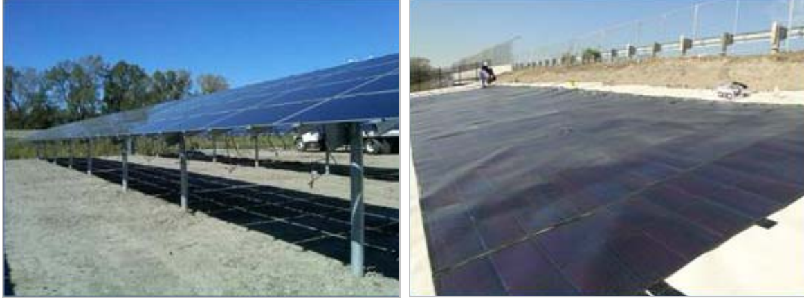
Figure 7: Rigid First Solar panels (left) and flexible Xunlight Corporation solar panels (right) installed along I-280 in Toledo, OH
